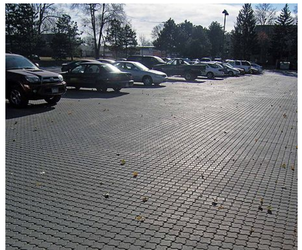
Example of a new retrofit permeable parking lot at the University of Minnesota
