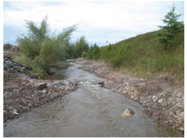
Stormwater step pool. Courtesy of Limnotech.
