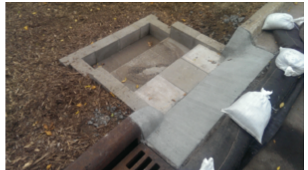
Modular Block Sediment Trap for pretreatment.
