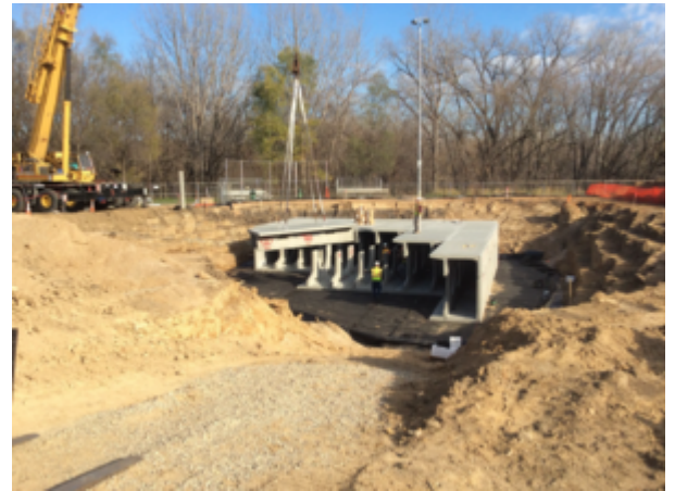
StormTrap underground storage vault for water stormwater reuse as irrigation.
