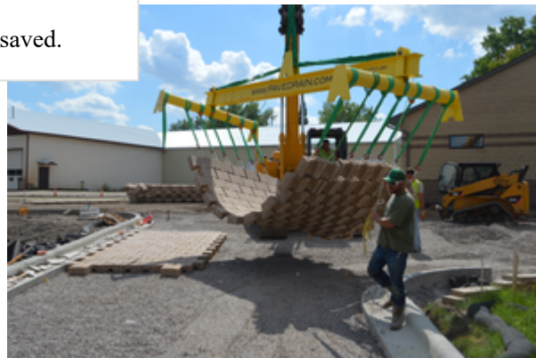
Permeable Pavers at Ramsey Washington Metro Watershed District. Photo Courtesy of Paige Ahlborg
