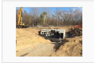
StormTrap underground storage vault
