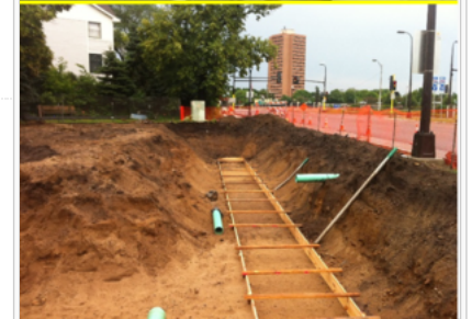
Partial excavation for retaining wall, infiltration basin is not excavated (top), retaining wall constructed, infiltration basin is fully excavated and has infiltration media in place (bottom). Photo courtesy of Barr Engineering.
