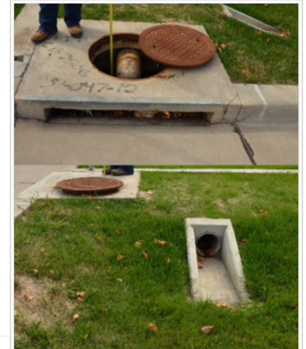
Pretreatment inlet structure to dry swale with check dam contains sump and skimmer (top), dry swale with check dam inlet pipe, downstream of inlet structure (bottom). Photos courtesy of Barr Engineering.
