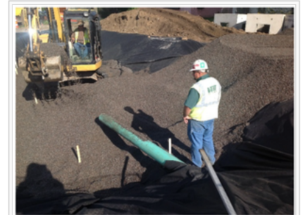
Infiltration media being placed in infiltration area with tracked backhoe. Photo courtesy of Barr Engineering.
