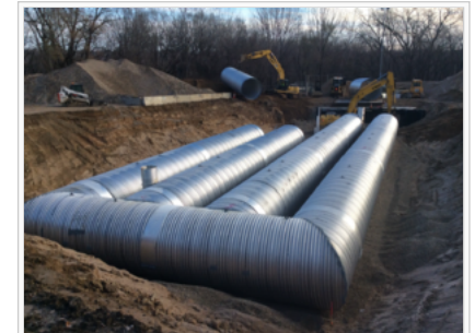
Underground TrueNorthSteel infiltration system in native sandy soils
