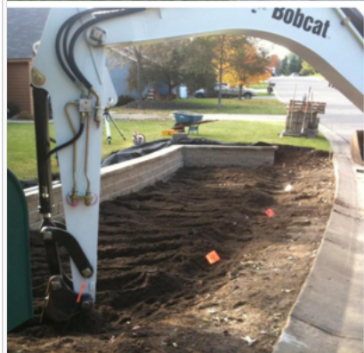
Example of subsoiling and incorporation of compost and sand. Note the equipment is kept out of the practice.
