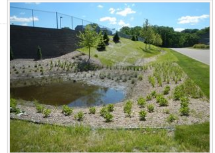
Example of a failing bioinfiltration system. Failure was due to clogging of the media surface by incoming sediment.
