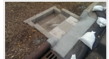
Modular Block Sediment Trap for pretreatment.
