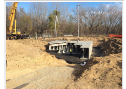
StormTrap underground storage vault for water stormwater reuse as irrigation.
