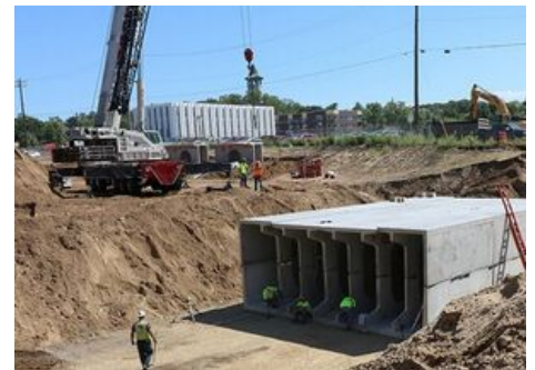
A 207,000-gallon cistern was constructed underneath the stormwater park biofiltration basin to store filtered runoff for eventual reuse.
