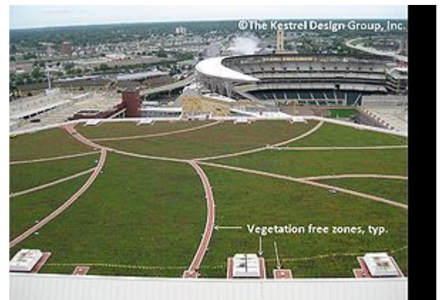
Green roof on the Target Center in Minneapolis Minnesota. Note the vegetation free zones. Image Courtesy of The Kestrel Design Group, Inc.
