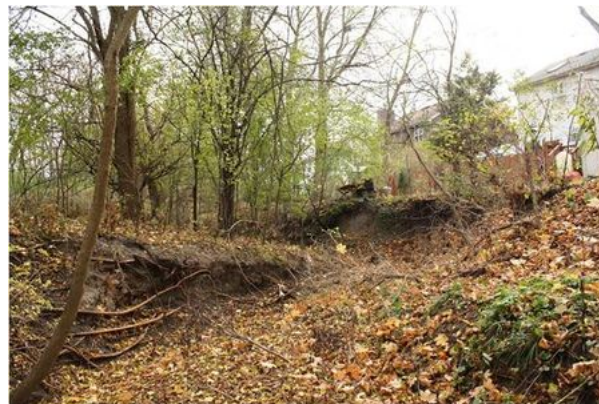
Eroded and failing structure banks contributing to sediment and nutrient loads along Carpenter Creek.
