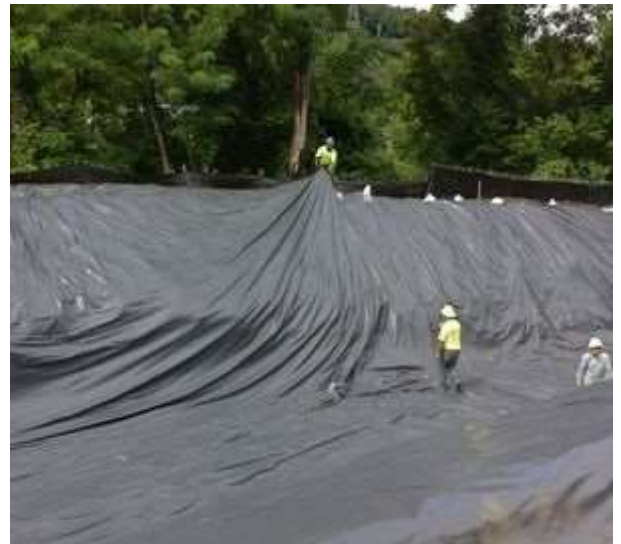
Example of an impermeable liner for a stormwater best management practice. Source: Philadelphia Water (PWD) Stormwater Management Guidance Manual ( https://www.pwdplanreview.org/manual/chapter-4/4.12-outlet-controls ).
