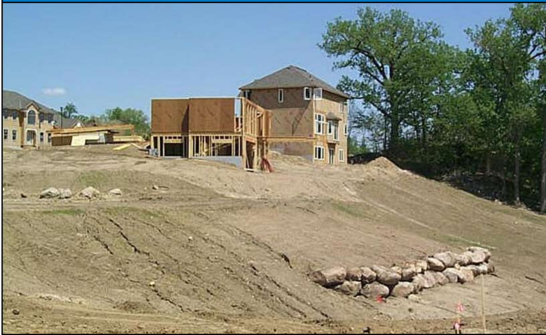
Figure 2.3 Uncontrolled Construction Erosion
