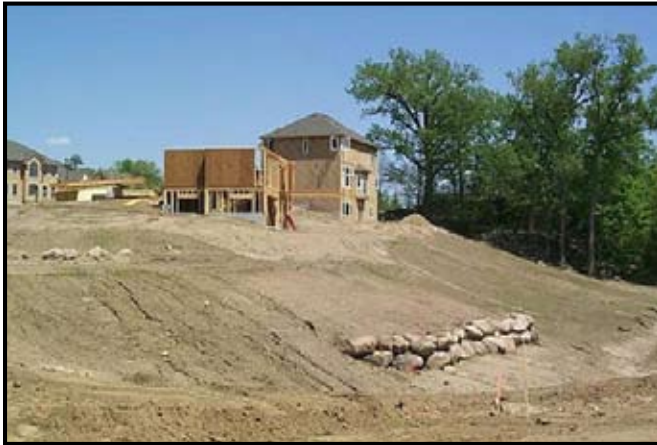
Site without temporary sediment control
