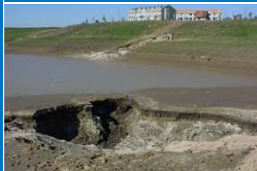
Figure 13.2 Collapsed Karst Feature
