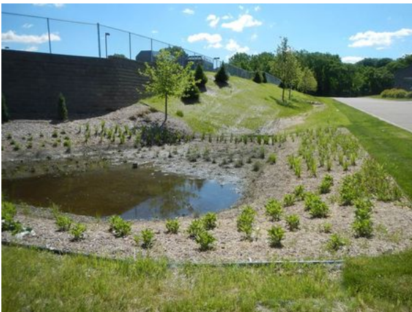
Ponded water in an infiltration practice may be an indicator of compacted soils.
