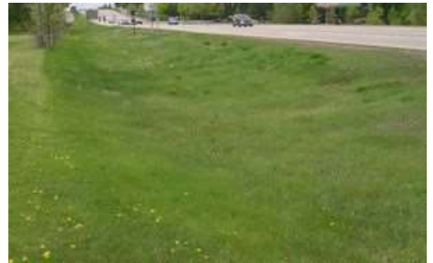
Photo of a dry swale. Courtesy of Limnotech.
