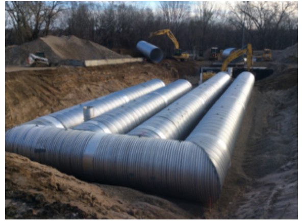
Underground TrueNorthSteel infiltration system in native sandy soils
