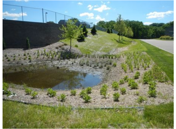
Example of a failing bioinfiltration system. Failure was due to clogging of the media surface by incoming sediment.
