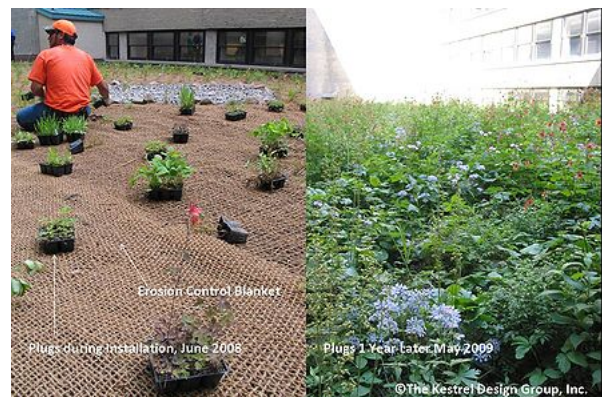
Erosion control blanket and native plant plugs at Minneapolis City Hall Green Roof, Minneapolis, MN. Image courtesy of The Kestrel Design Group, Inc.
