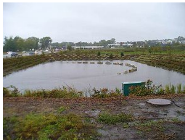
Iron enhanced sand filter basin, Maplewood, MN. If this sand filter is performing properly, it will drain within 48 hours. Photo courtesy of Barr Engineering.
