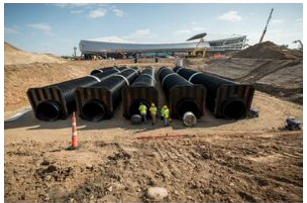
Underground storage tanks
