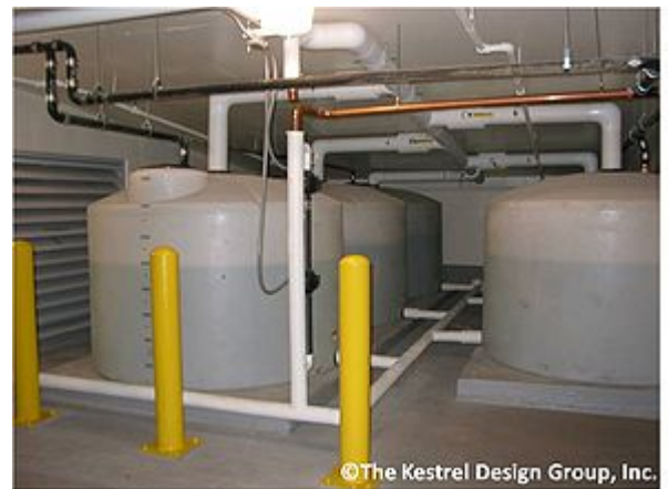
Minneapolis Central Library cisterns in an underground parking garage. The cisterns harvest stormwater runoff for irrigation
