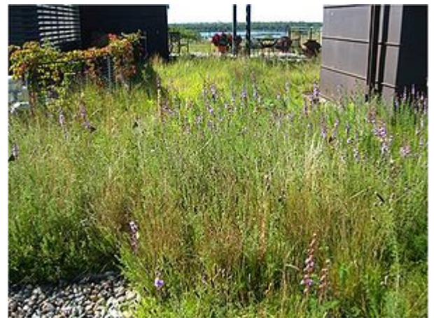
Edgewater green roof, illustrating the use of native prairie plants and vines (background) Image Courtesy of The Kestrel Design Group, Inc.
