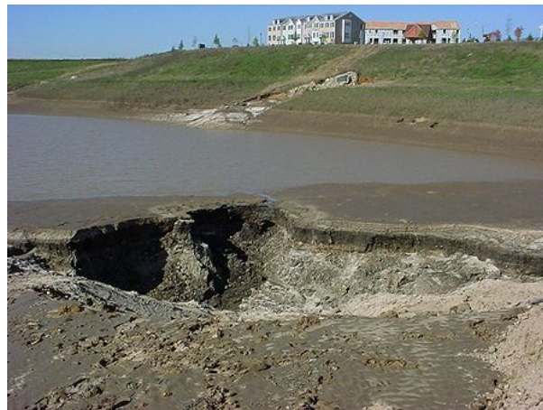
A collapsed karst feature where a stormwater pond previously existed. The site was in Woodbury, Minnesota.
