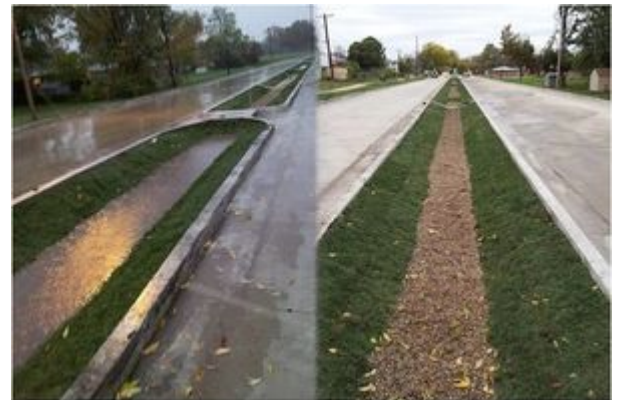
View of an installed dry swale during a rain event and during dry conditions.
