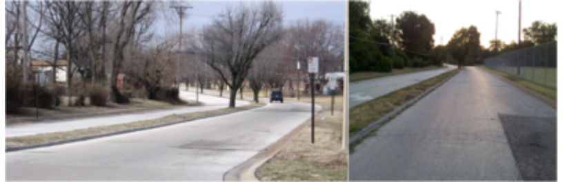
Views of International Plaza Drive and pavement failure and repairs.
