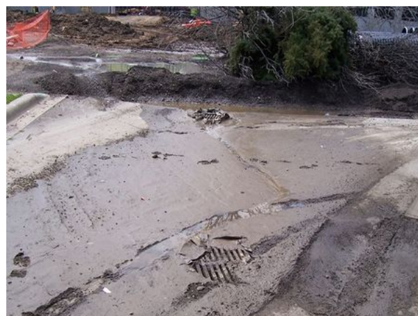
Example of poorly managed construction site. Runoff from the street will be heavily laden with sediment and include pollutants attached to the sediment.
