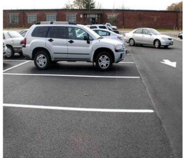
Photo illustrating porous asphalt. Porous asphalt is standard hot-mix asphalt that allows water to drain through it.
