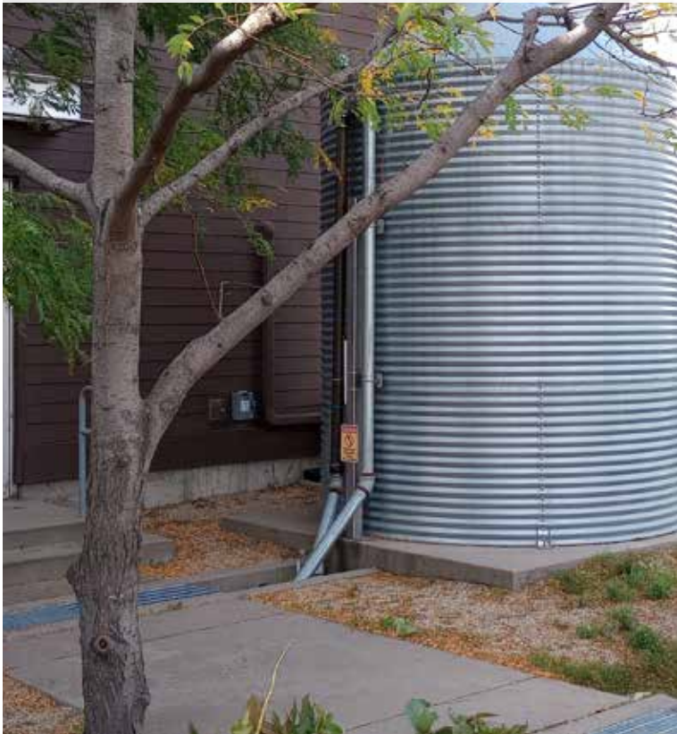
The cistern at the Mississippi Watershed Management Organization (MWMO) office collects rainwater from the building's roof to water the trees in the trench system. Photo courtesy of MWMO.
