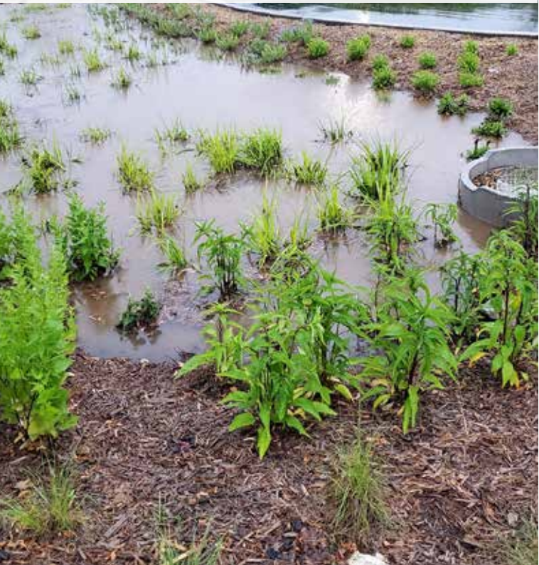
This new bioretention facility in Eagan is capturing and holding stormwater from the adjacent parking lot during this rainstorm, functioning as intended. Photo courtesy of Brendan Dougherty, Barr Engineering Co.
